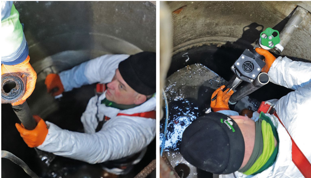
Fig. 2: Removal of the old sump internals due to corrosion and replacement with the new Installation Set.
