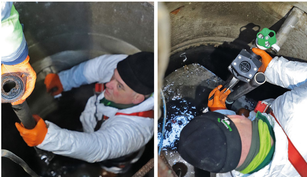
Fig. 2: Removal of the old sump internals due to corrosion and replacement with the new Installation Set DN 40
